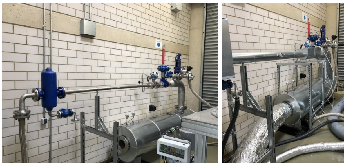
Figure 18: Steam control line prior to complete assembly and insulation (l.h.s.) and after complete assembly (r.h.s.).
