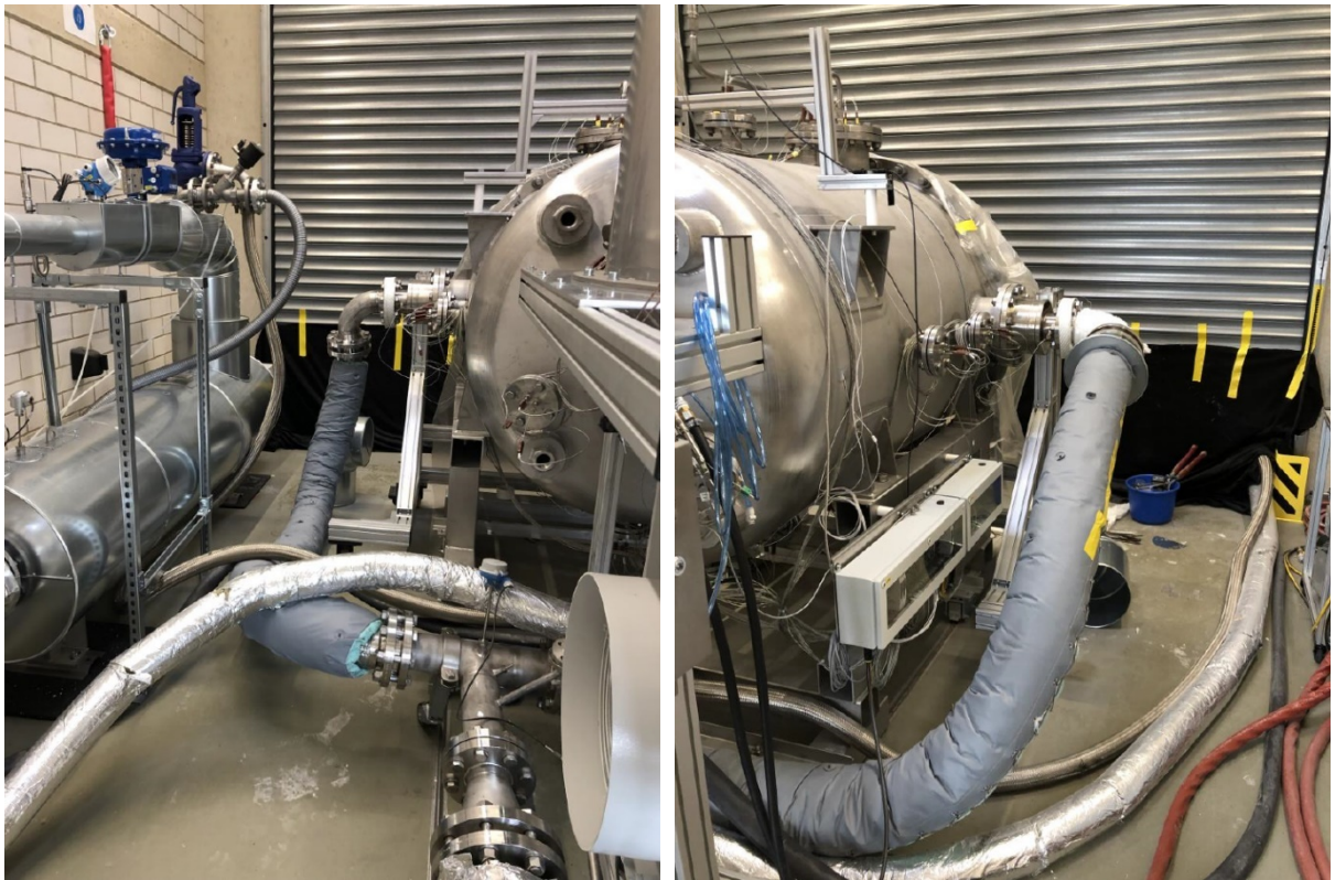
Figure 19: Steam feed from the superheater to the receiver manifold.
