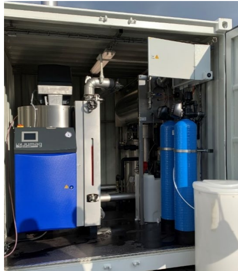
Figure 12: Representative example of steam generator.
