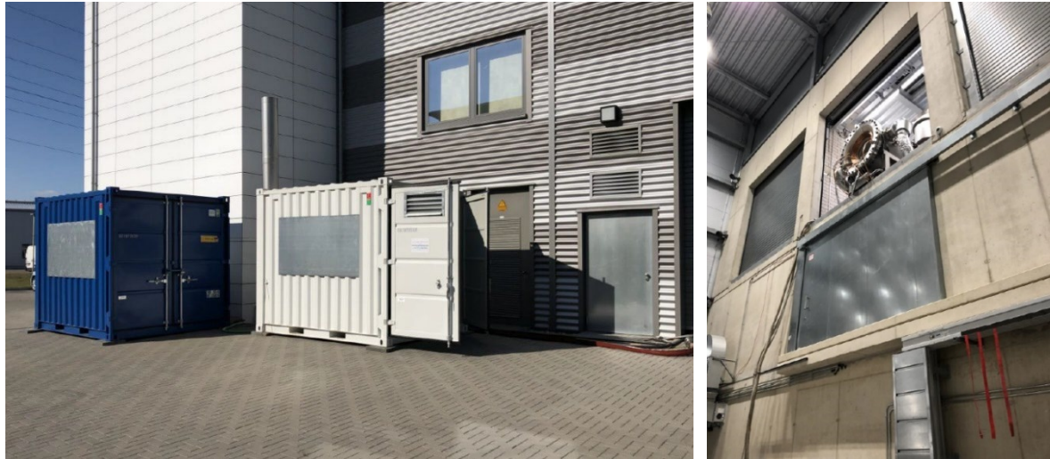
Figure 17: Steam generator situated outside of DLR Synlight building (l.h.s.). Steam hoses transporting the steam from the container to the inner test chamber (r.h.s.).
