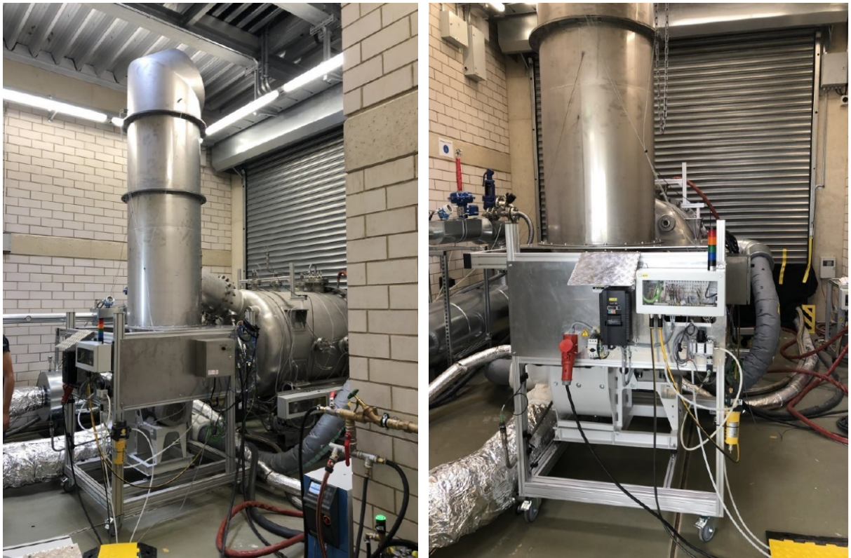
Figure 20: Steam cooling system with chimney (l.h.s.) and industrial blower (r.h.s.).
